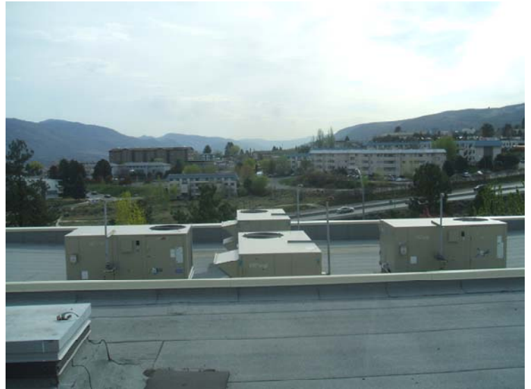
11. A-Block Addition RTUs.JPG
