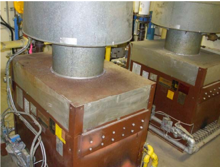
2. Boiler Plant B-1.JPG
