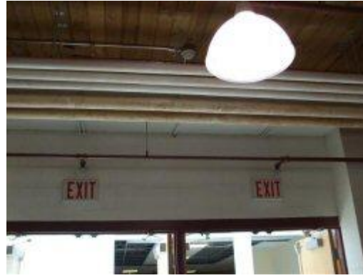
Figure 36: Burnt-Out Exit Signs in OM
