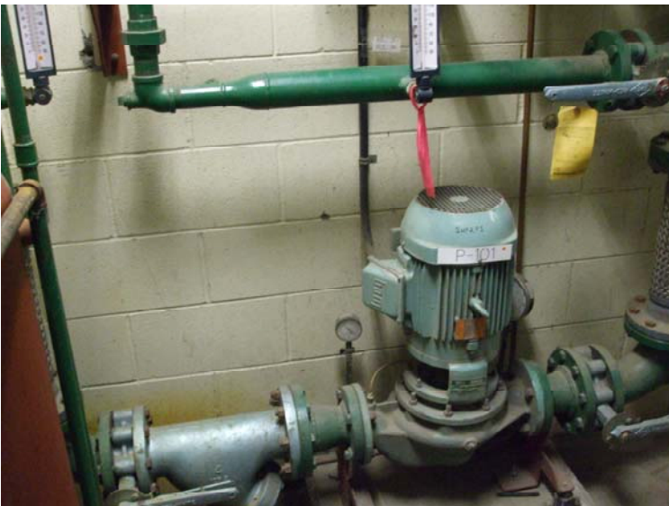
3. Heat Pump Loop Pump P-101.JPG
