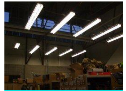
Figure 30: TT Equipment Room
