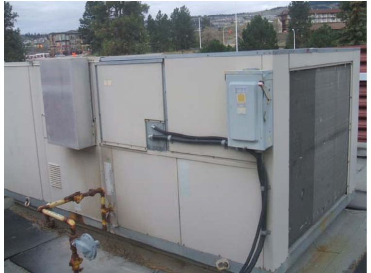
5. Theatre Rooftop Unit.JPG
