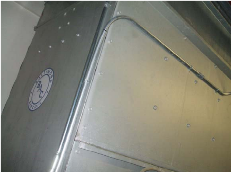
5. Cooling Tower (Typical of 2).JPG
