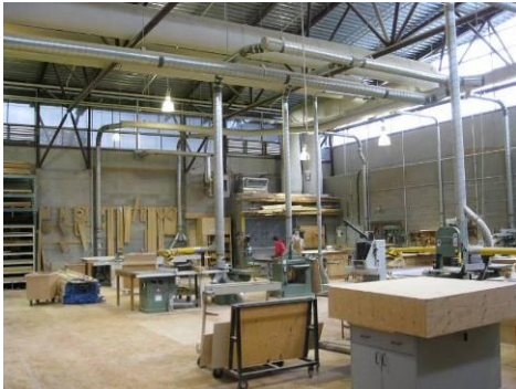
Figure 50: Woodshop Exhaust Ducting
