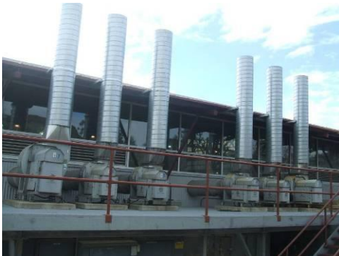
Figure 48: Welding Booth Exhaust Fans
