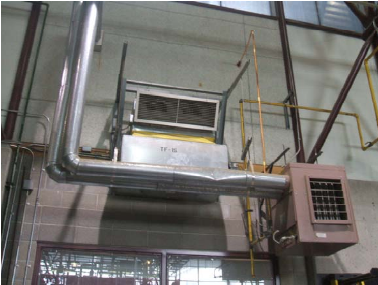
8. Typical Transfer Fan.JPG
