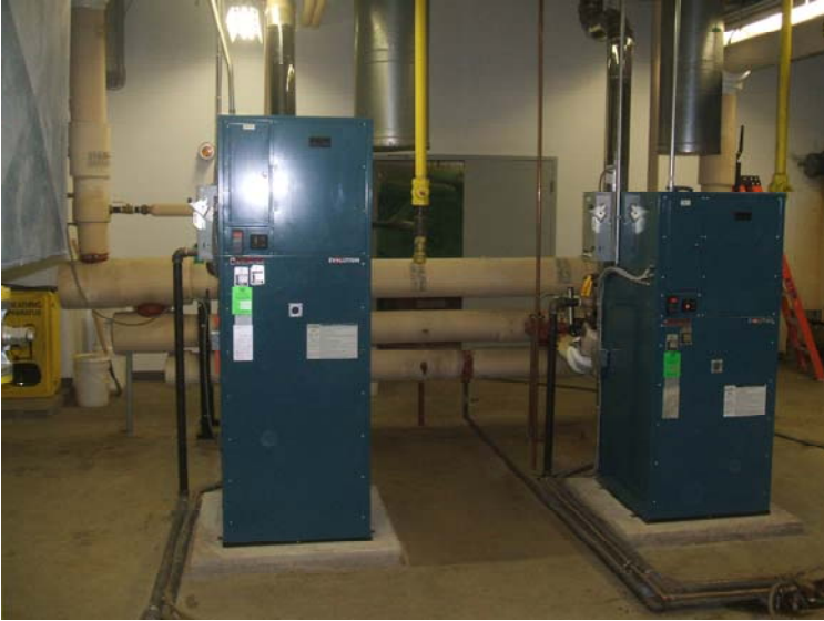
1. Heating Plant A-Block.JPG
