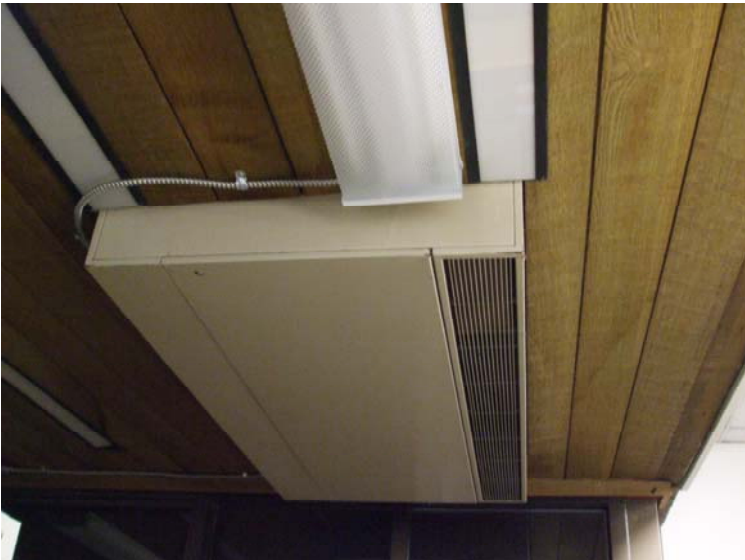
3. Entrance Forced Flow heaters.JPG
