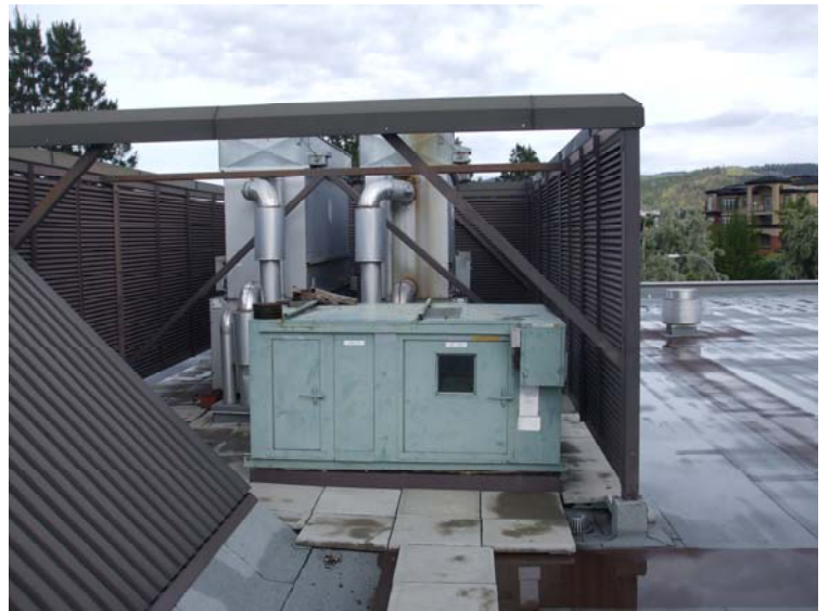
5. SF1, AF2 and Cooling Towers.JPG
