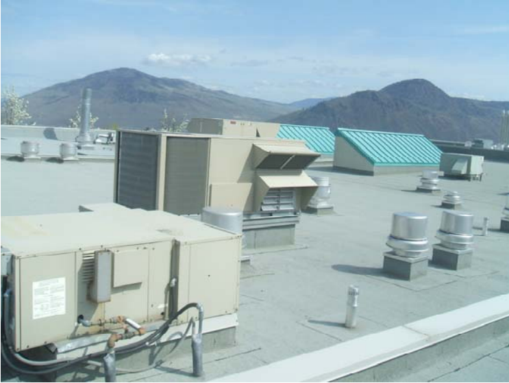
13. C-Block RTUs and Exh Fans.JPG
