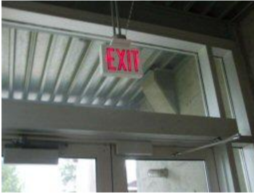
Figure 35: LED Exit Sign In TT
