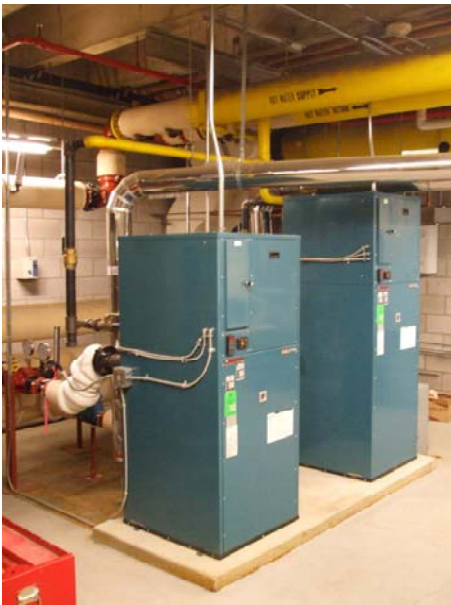
2. Heating Plant B-Block.JPG
