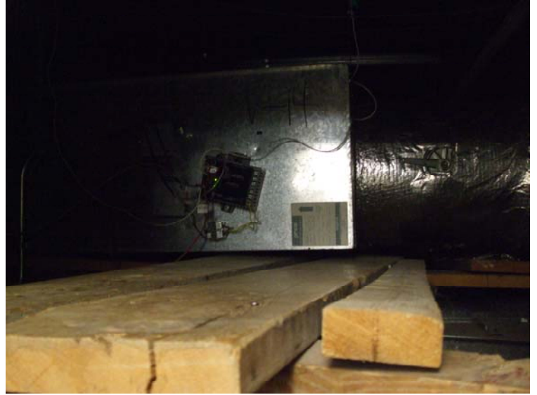
4. Typical VAV Bypass Box.JPG
