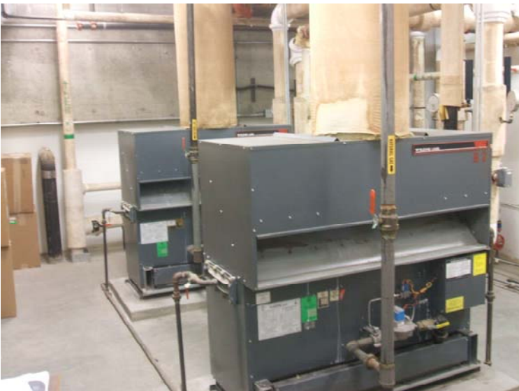
3. Heating Plant C-Block.JPG
