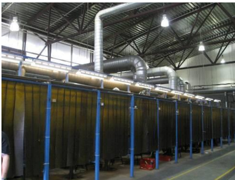
Figure 47: Arc Welding Booths
